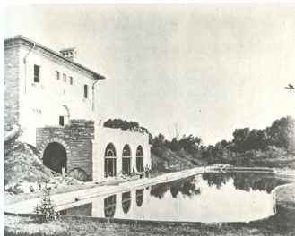
East side of Marland Mansion during construction, showing the already completed Swimming Pool
